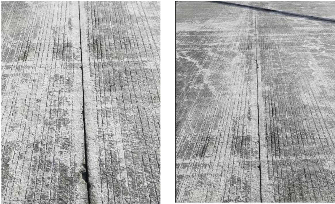
Figure 4. Disruption of joint edges
