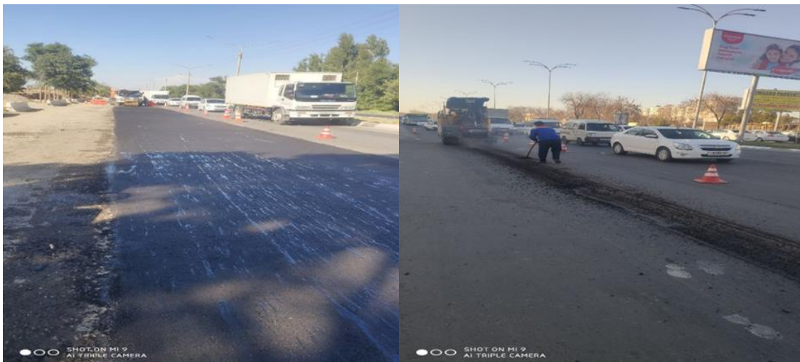
Figure-7. Condition of road markings and guardrails on the road section under repair.
