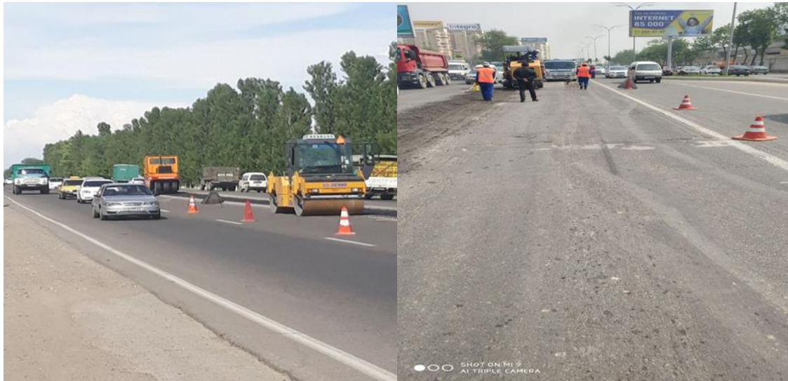
Figure-1. In real conditions, road signs and guardrails are installed on the section of road being repaired.
