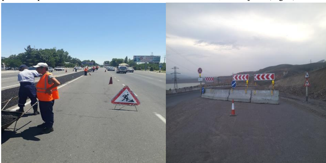
Figure-5. Condition of road markings and guardrails on the road section under repair.
