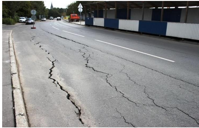
Picture 2. Longitudinal cracks
