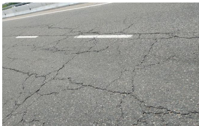
Picture 6. Y and X-shaped cracks
