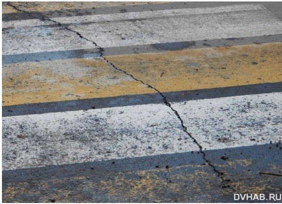
Picture 1. Transverse cracks
