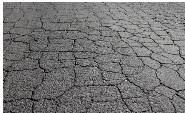
Picture 4. A network of cracks
