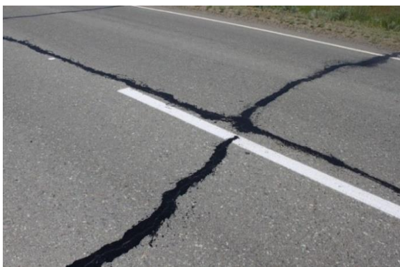
Picture 3. Both transverse and longitudinal cracks
