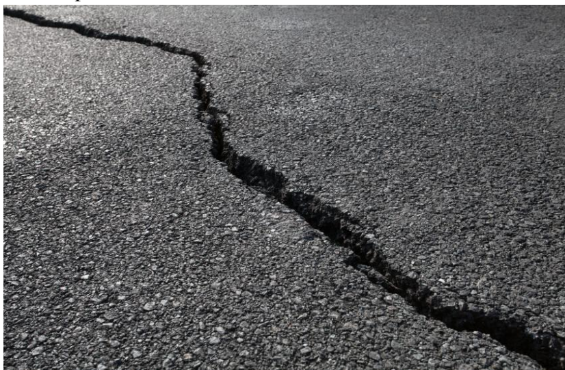
Figure 1. Cracks on roads in hot climates.
