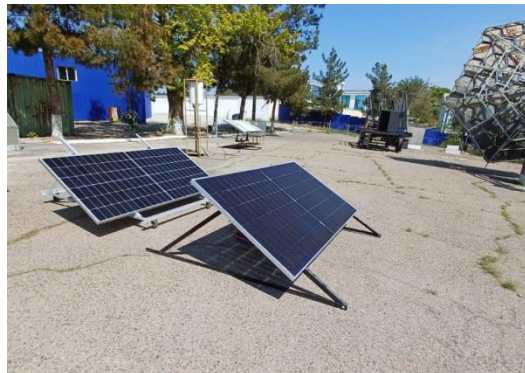
Figure 3. The general arrangement of solar panels.
