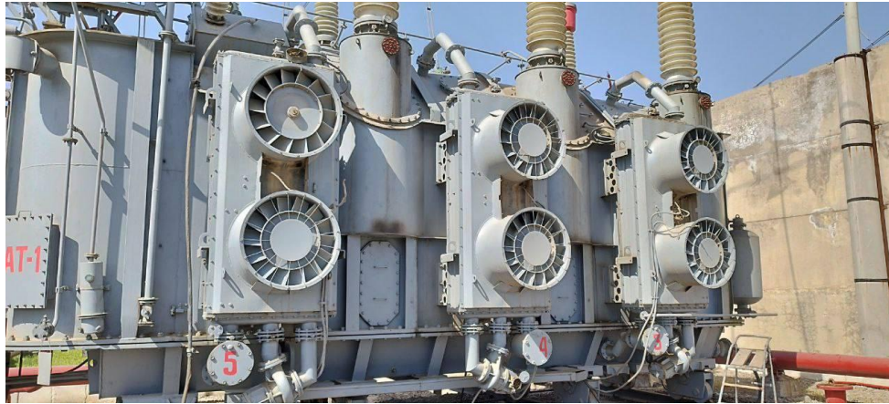
Fig. 1. Power autotransformer PS Yuksak.
