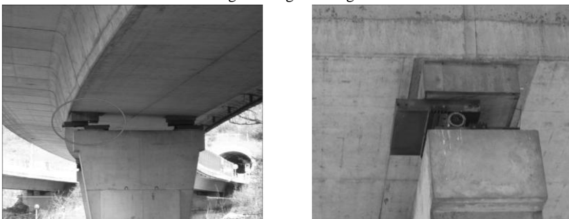
Damage to hinge bearing elements
