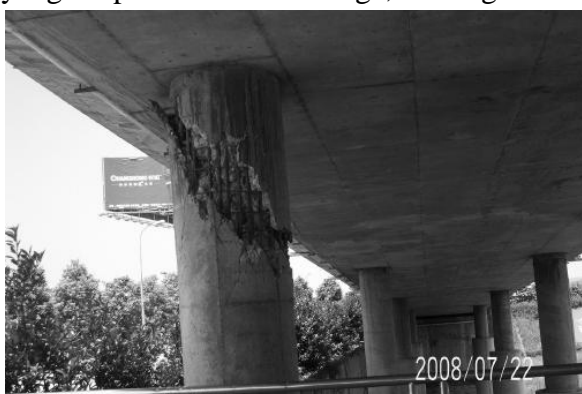
Mianyang Airport Terminal Bridge, bearing shear failure
