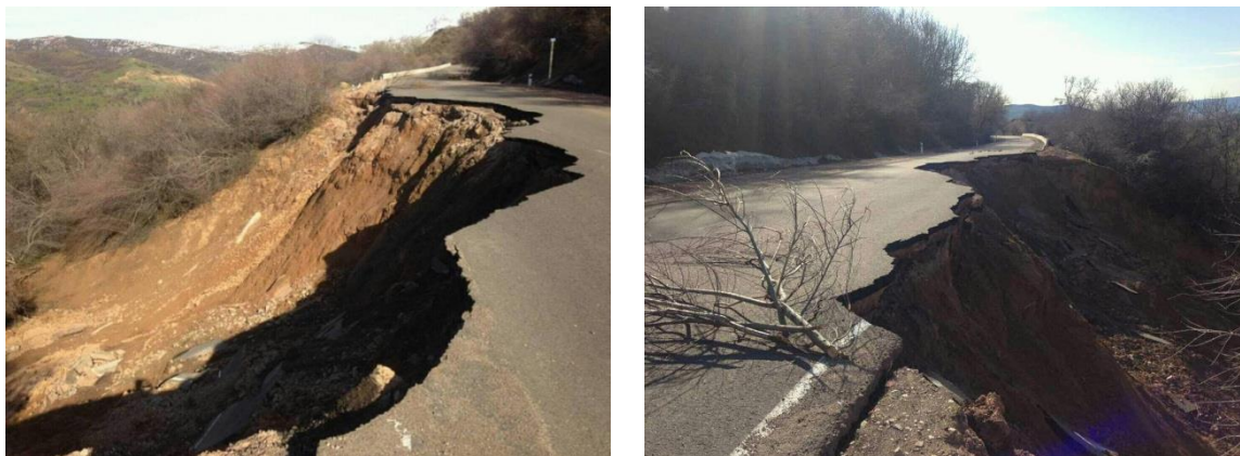
Figure 1. Landslides on the area of the road
